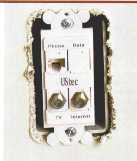
Interface with this. Really. This tech port is set up to handle phone and video. Other options are myriad, and a Decora-style plate finishes off the installation.
